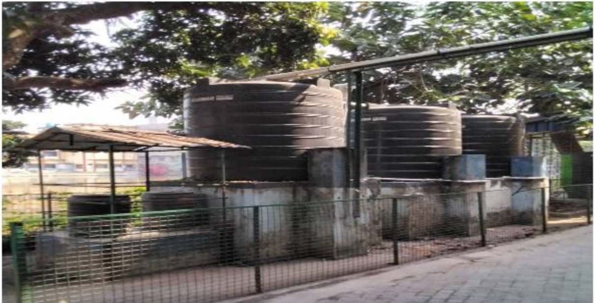
Fig.8: Rain water collect storage tank
