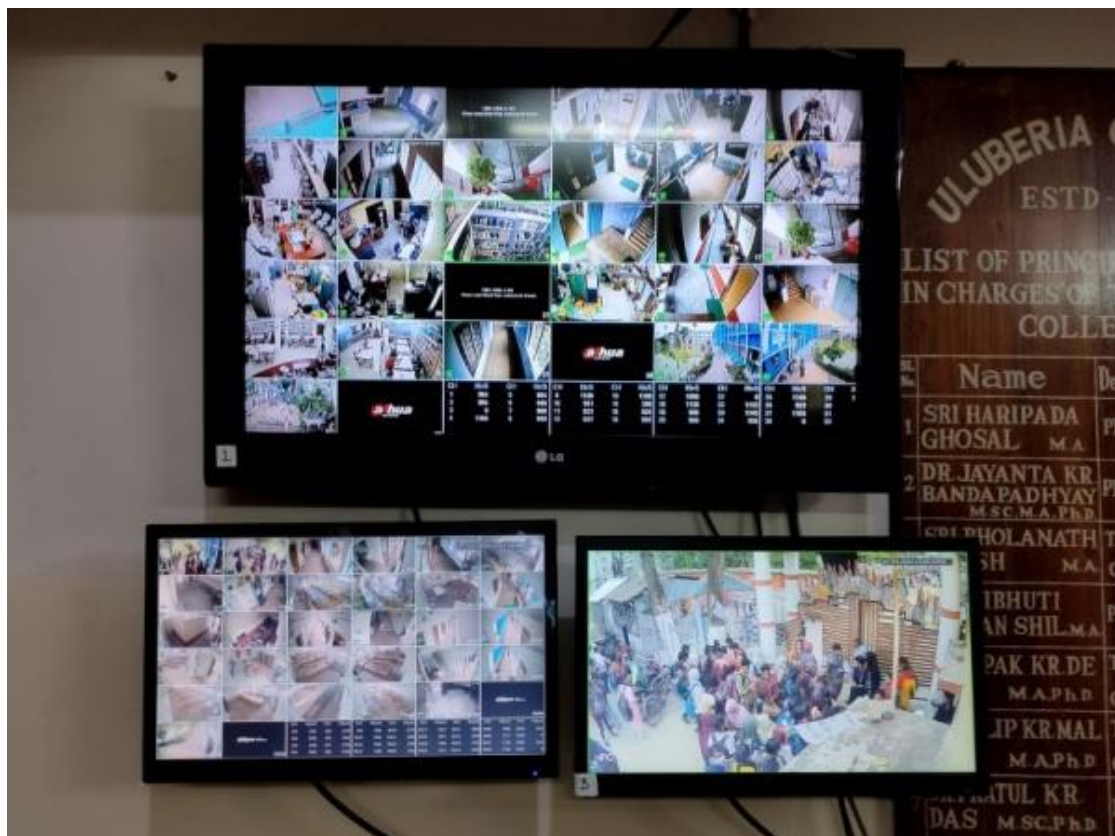
CC TV Control panel installed at Principal's Room
